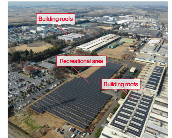
Panoramic view of the PV power generation system at the Moka site
