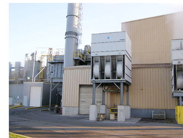
Closed-loop cooling water systems
