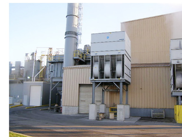
Closed-loop cooling water systems
