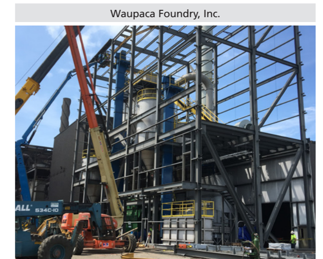
Sand recycling system adopted by Plant 5
