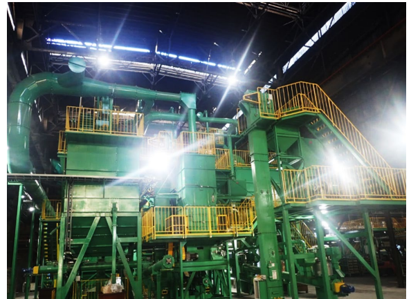
Sand recycling equipment
