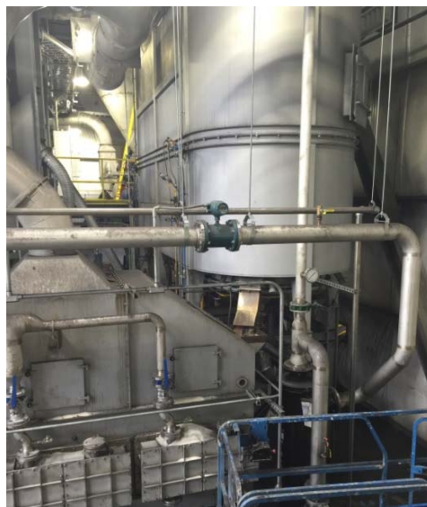
Sand recycling system introduced at Plant 5
