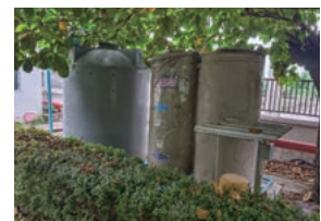
Tank to store treated rainwater
