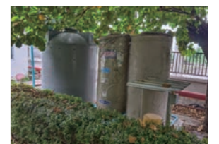
Tank to store treated rainwater
