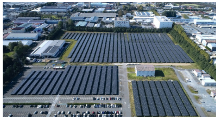
On-site solar power generation facilities for in-house consumption, installed at the Kumagaya district
